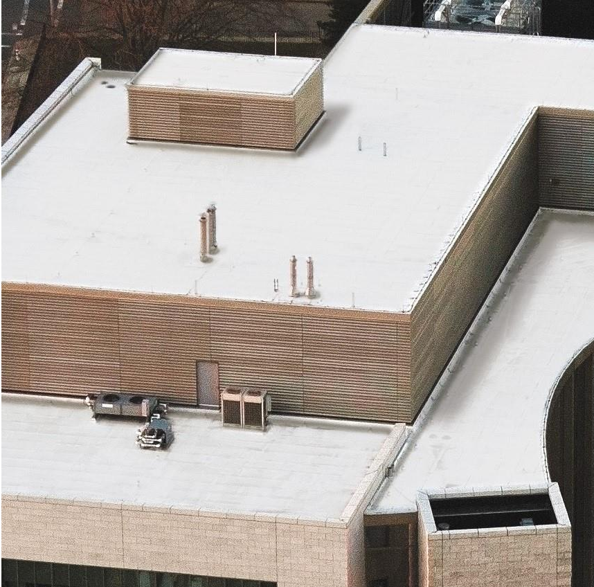
Singly ply, TPO membrane mechanically fastened and representative of 45, 60, and 80 mil thicknesses
